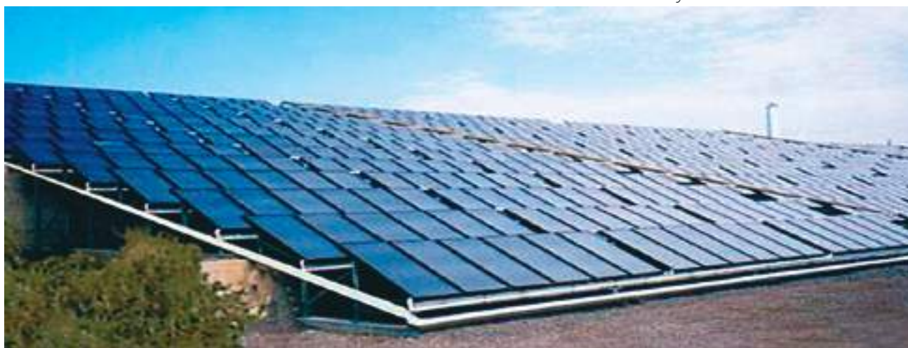
SARANTISS.A., 1999-Solar Air -Conditioning 700kw
